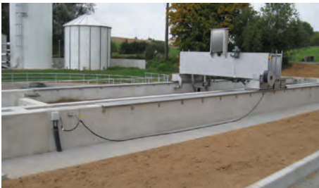
▪ HIK Sandfangräumer / HIK sand trap scraper
